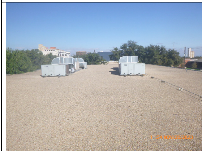
View of The HVAC Units on the Roof (Photograph 21)
