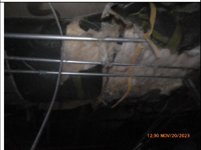
View of the Non-ACM HVAC Duct Insulation (Photograph 12)
