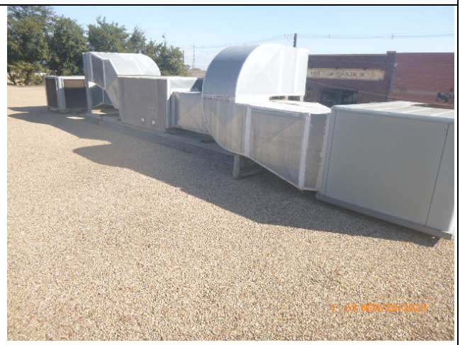
Close View of the HVAC Units (Photograph 22)
