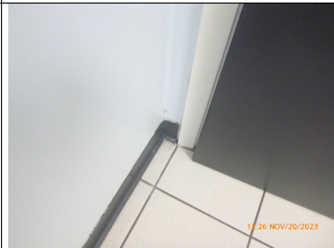
Close View to the Ceramic Floor Tile and the Cove Base (Black) (Photograph 04)
