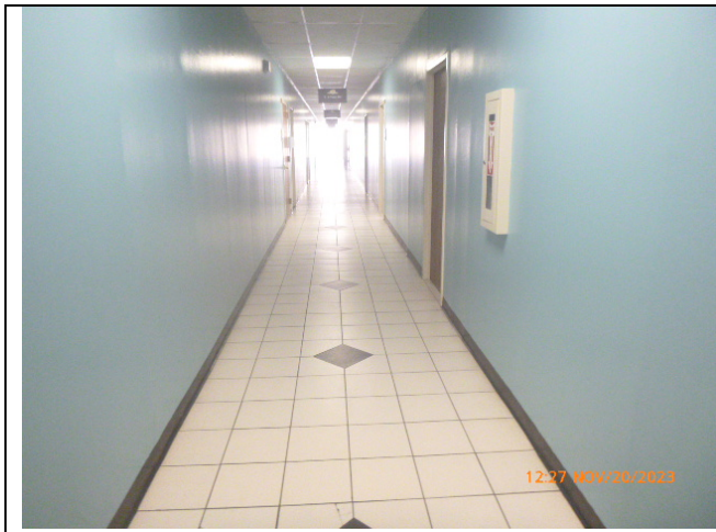
View of the Floor Ceramic Tile and the Drywall in the Hallway (Photograph 07)
